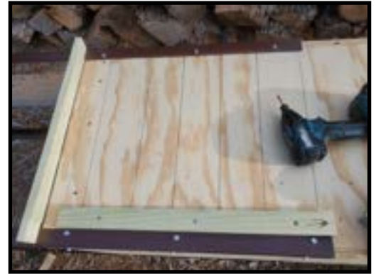
Figure 9 - Outside Vertical Cleat installed next to the Steel Leg and Outside Horizontal Cleat showing notches that will fit over the Steel Legs
